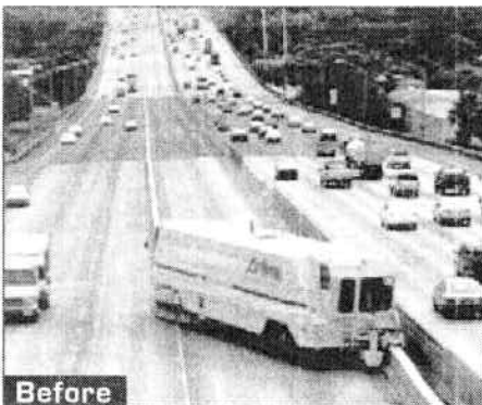
Barrier being transferred from the stored median position creating additional contraflow lanes - Honolulu, Hawaii
